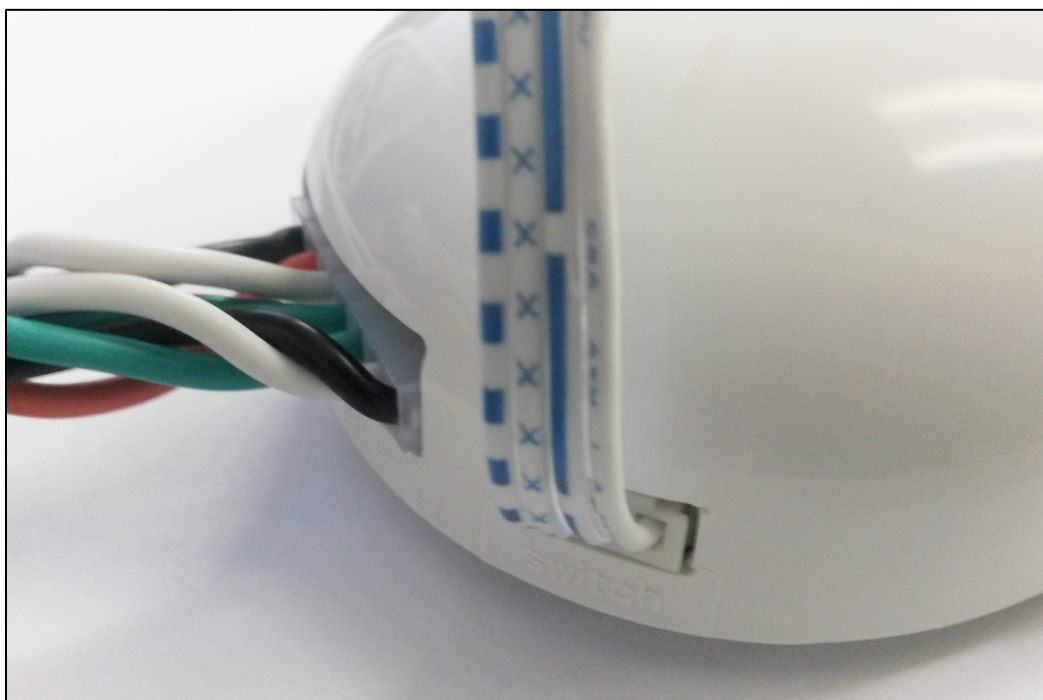
Dry Contact Wiring Harness connected to GC154
