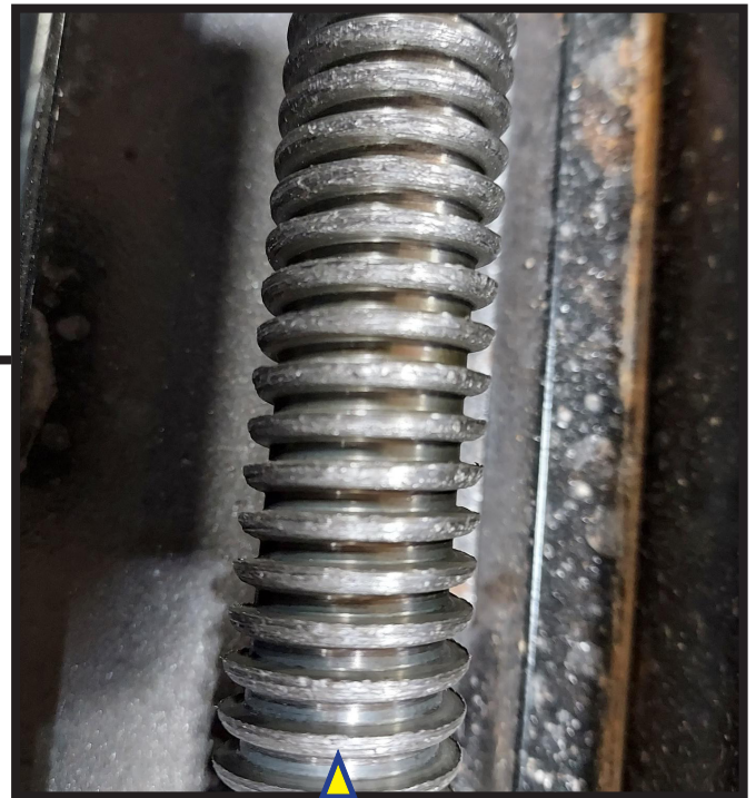
Damaged Screw Gear
