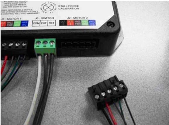
Motor connection at board
