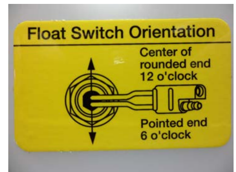
Figure 11 Label on side of vertical tank
