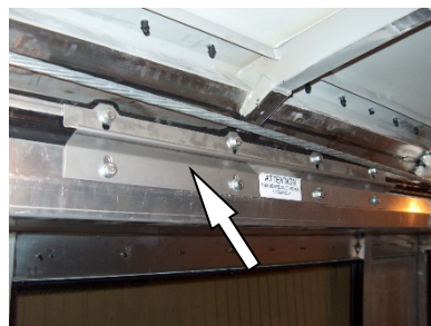
Interior roof hooks
